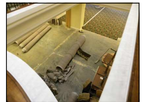
Under construction: This is a bird's eye view of the Avalon Dining Room as the new carpet was being installed last month.
